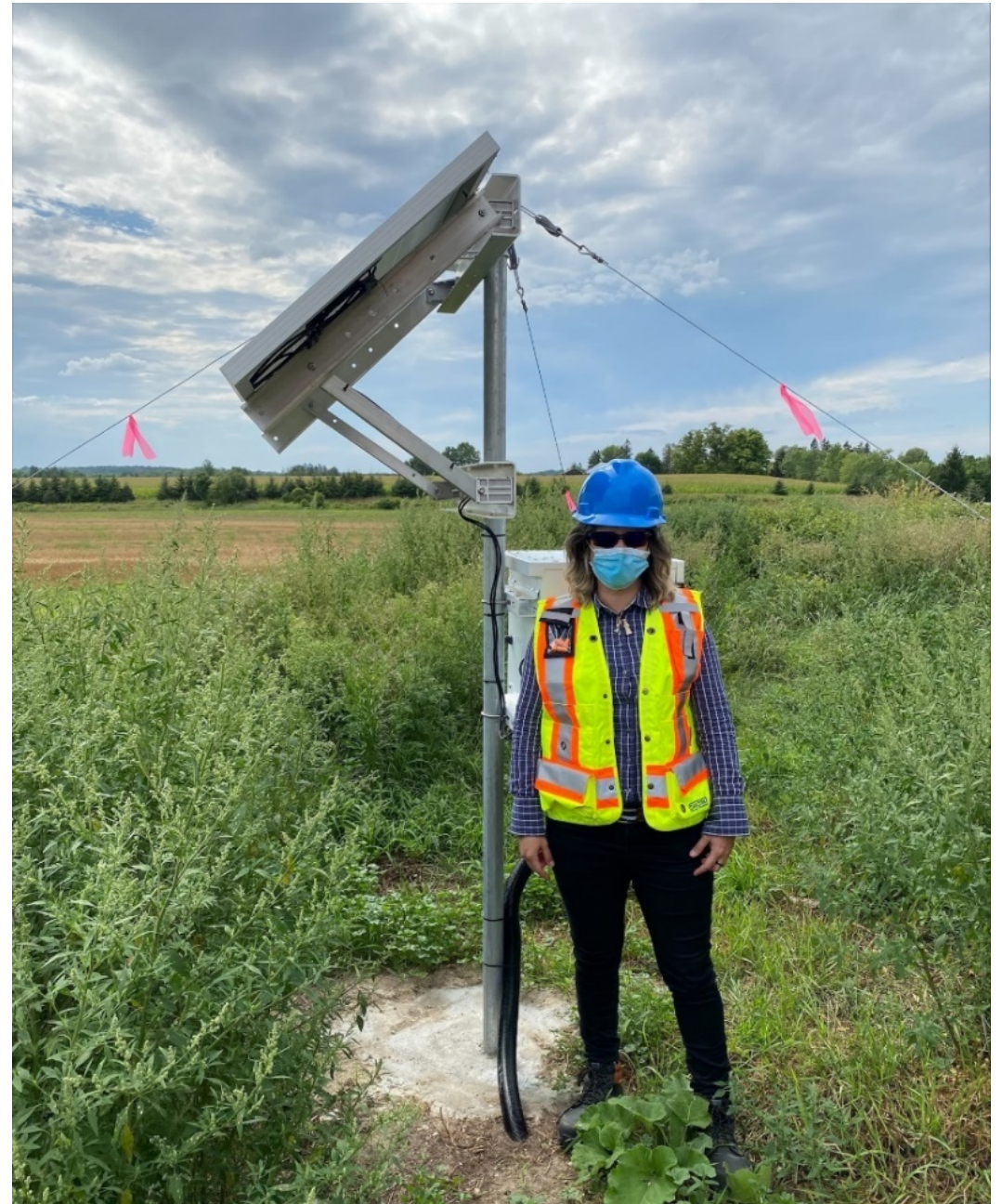
One of five microseismic monitoring stations installed in area
