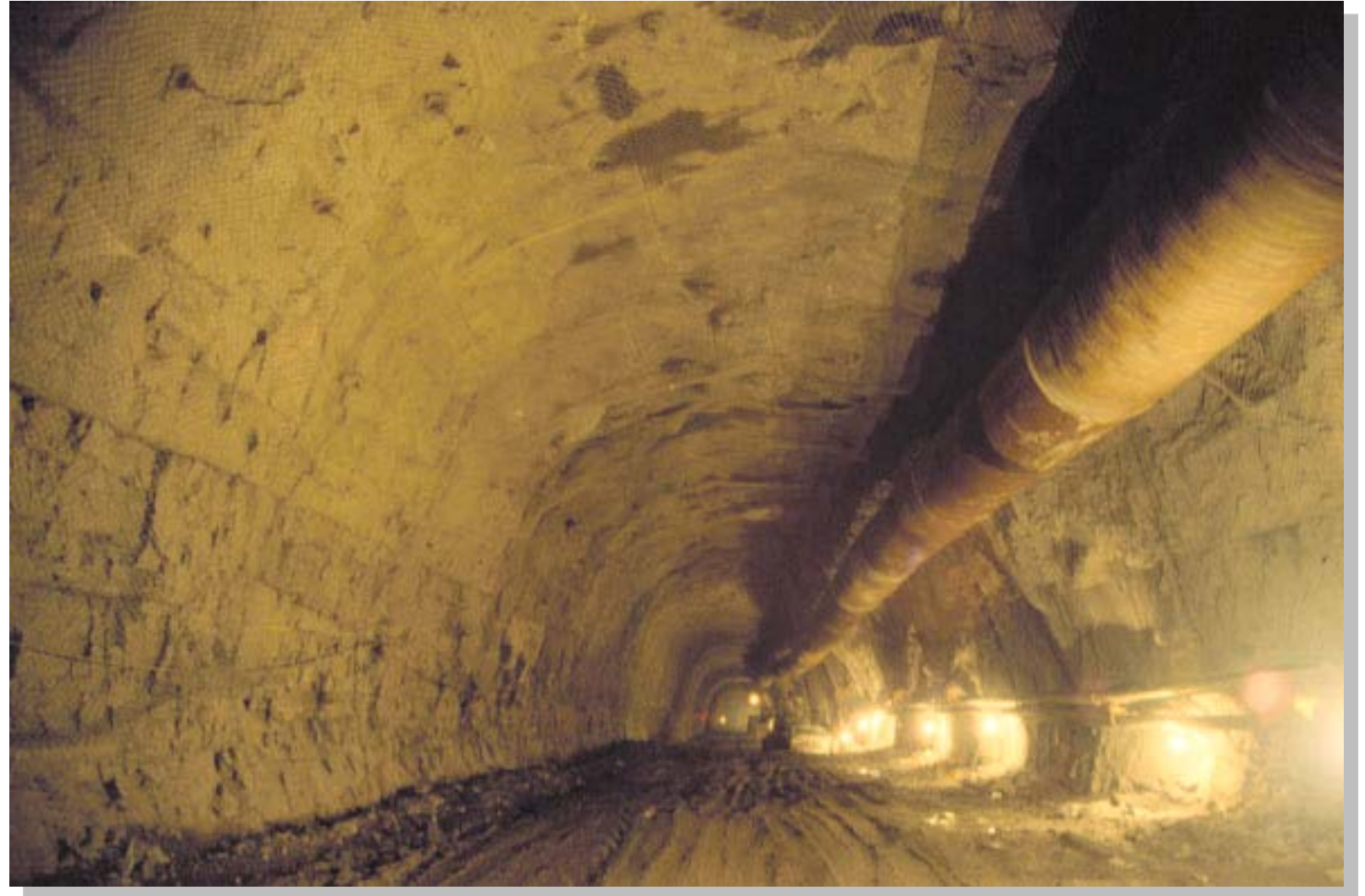
Darlington Intake/Discharge Tunnels (under Lake Ontario)
